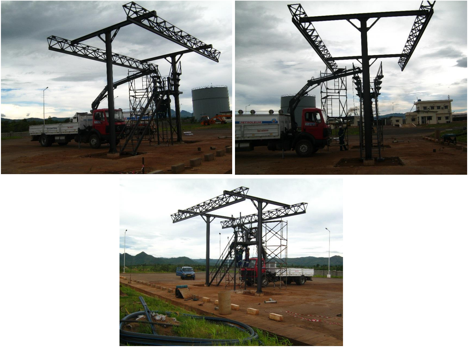
Figure 26 Fabrication and Installation of Fall Arrest Canopies at National Oil Company of Malawi
