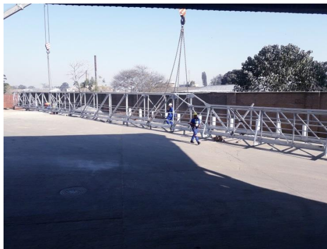
Figure 27 Construction and Erection of Conveyor Bridge Steel Structure at Bakhresa Factory Limbe 85m span
