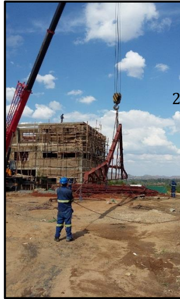
Figure 9 Fabrication and installation of Steel Roof Installation at AMITOF0 Care Centre in Chiladzulu
