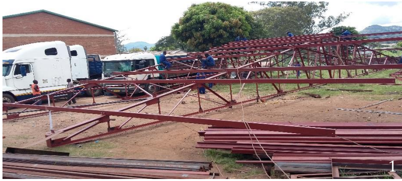
Figure 12 Above Fabrication of Trusses for Puma Filling Station Shop at our workshop in Blantyre
