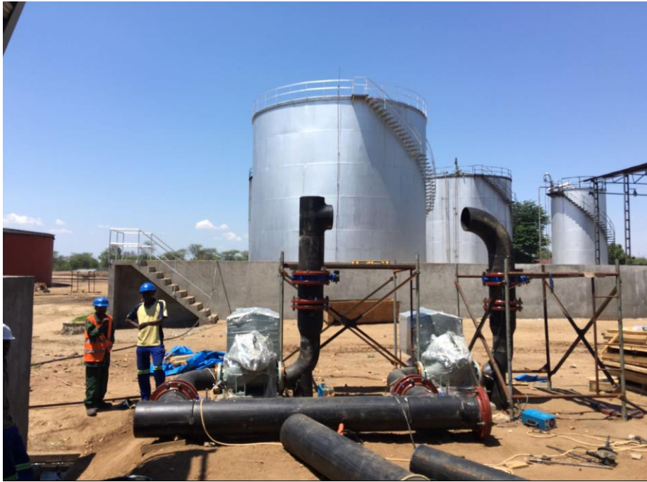
Figure 7 Presscane Chikwawa-Tanks and pipes
