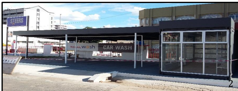
Figure 15 Above Fabrication and installation of Container Kiosk and Car Wash Bay in Blantyre
